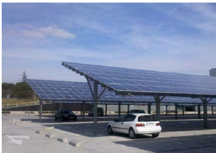
Ombrières photovoltaïques (©Hanjin)
